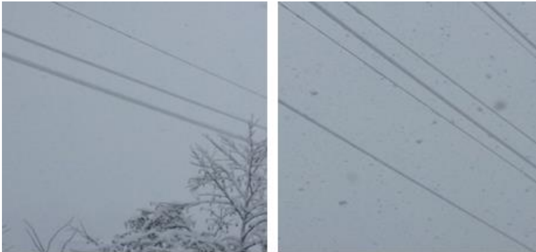
Figure 7 Ice Accumulation on Overhead Line Confirmed with Field Trip
