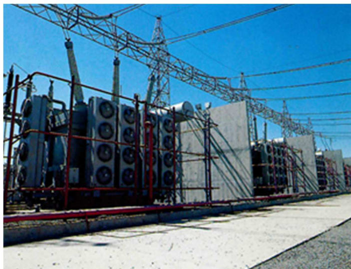
Figure 8. UHV-Power transformer substation
