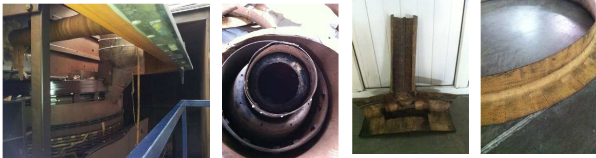
Fig.15. Photos of short circuit insulation components in this Case Study
