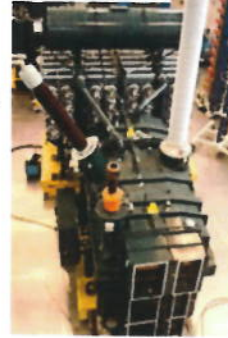
735 kV RIP bushing
