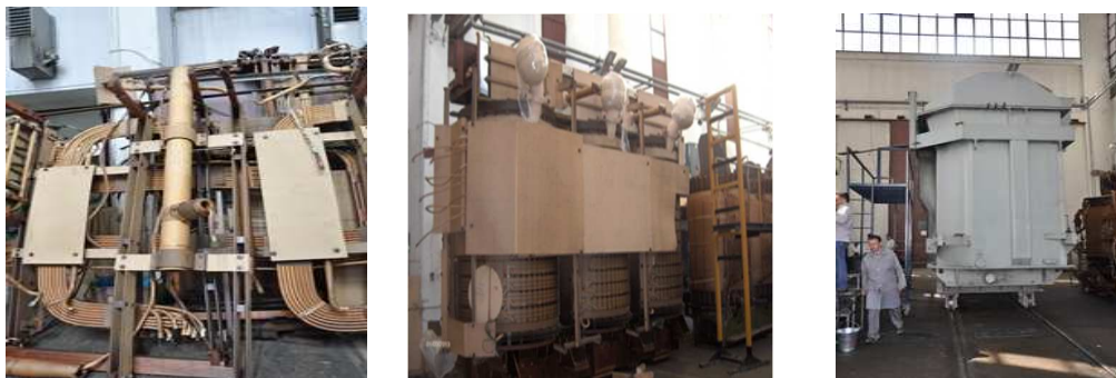
Figure 16. renewed connecting cables and upper insulation part, finished active part of transformer
